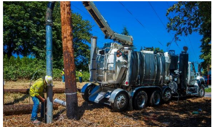
In 2016, we coordinated with Olympic on the work plan and safe construction practices to replace two pole structures in Newcastle.
