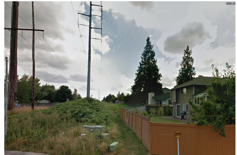
230 kV transmission line in Everett, WA
