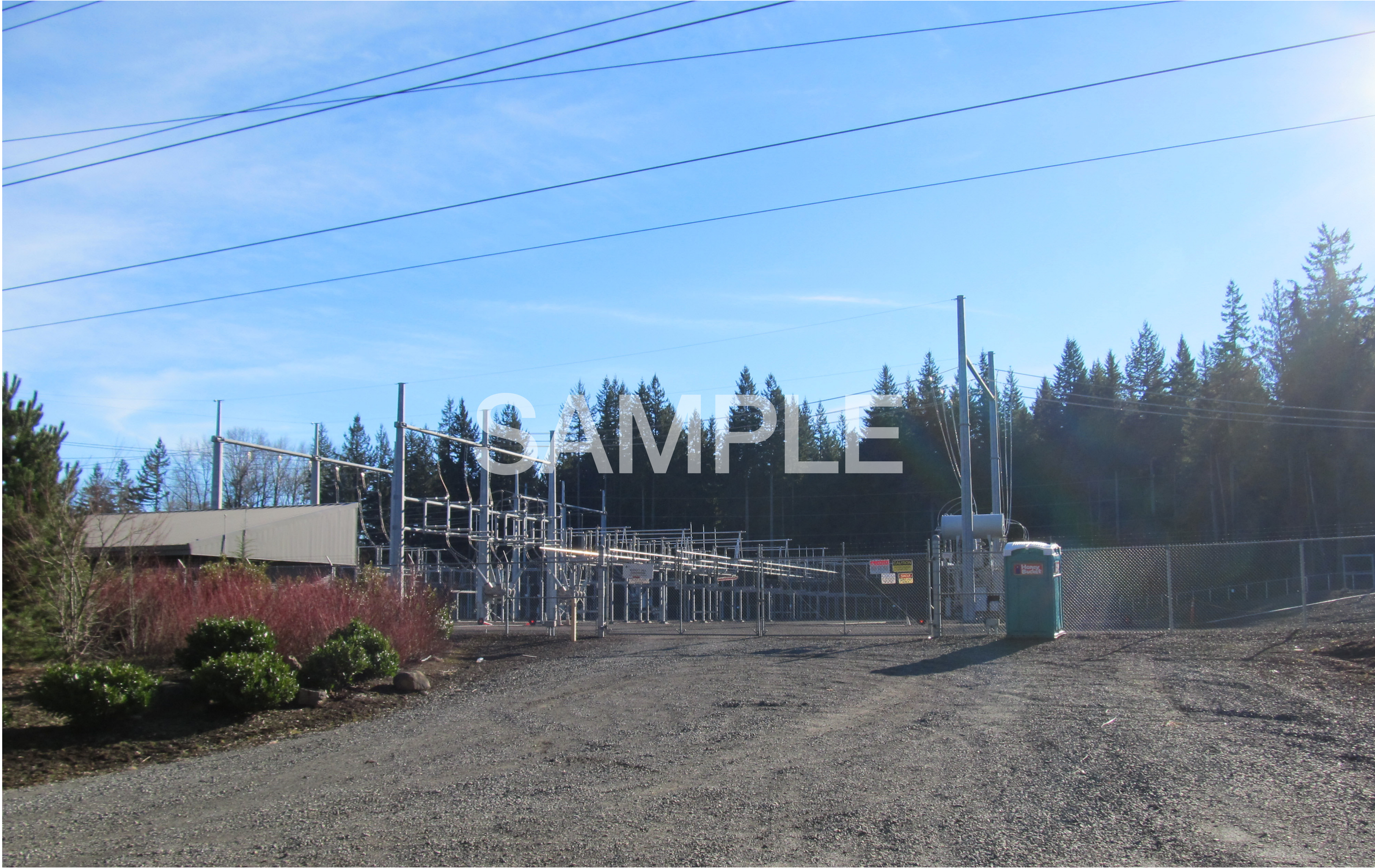
Novelty Hill 230 kV Substation
