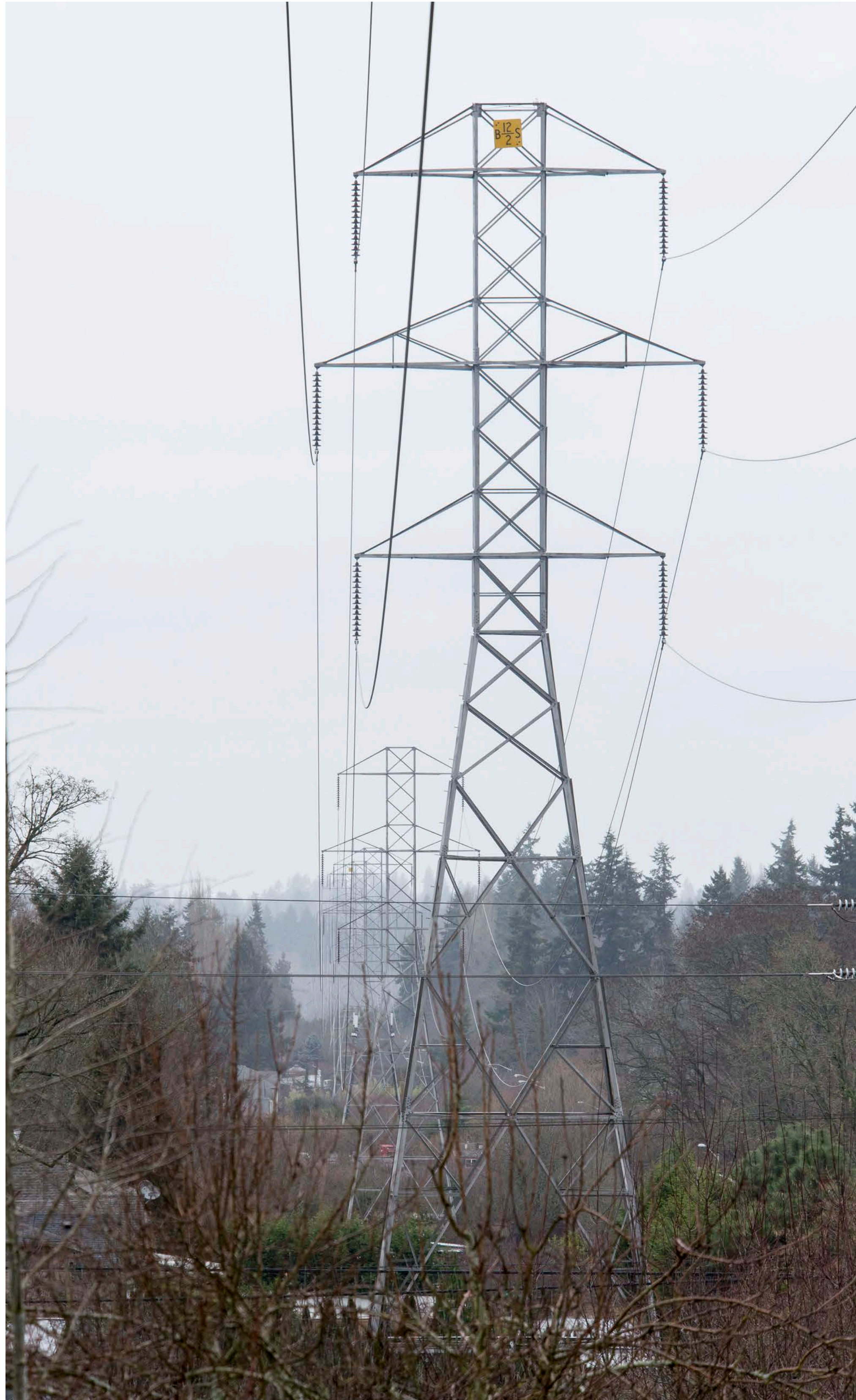
A Seattle City Light 230 kV transmission lines.
