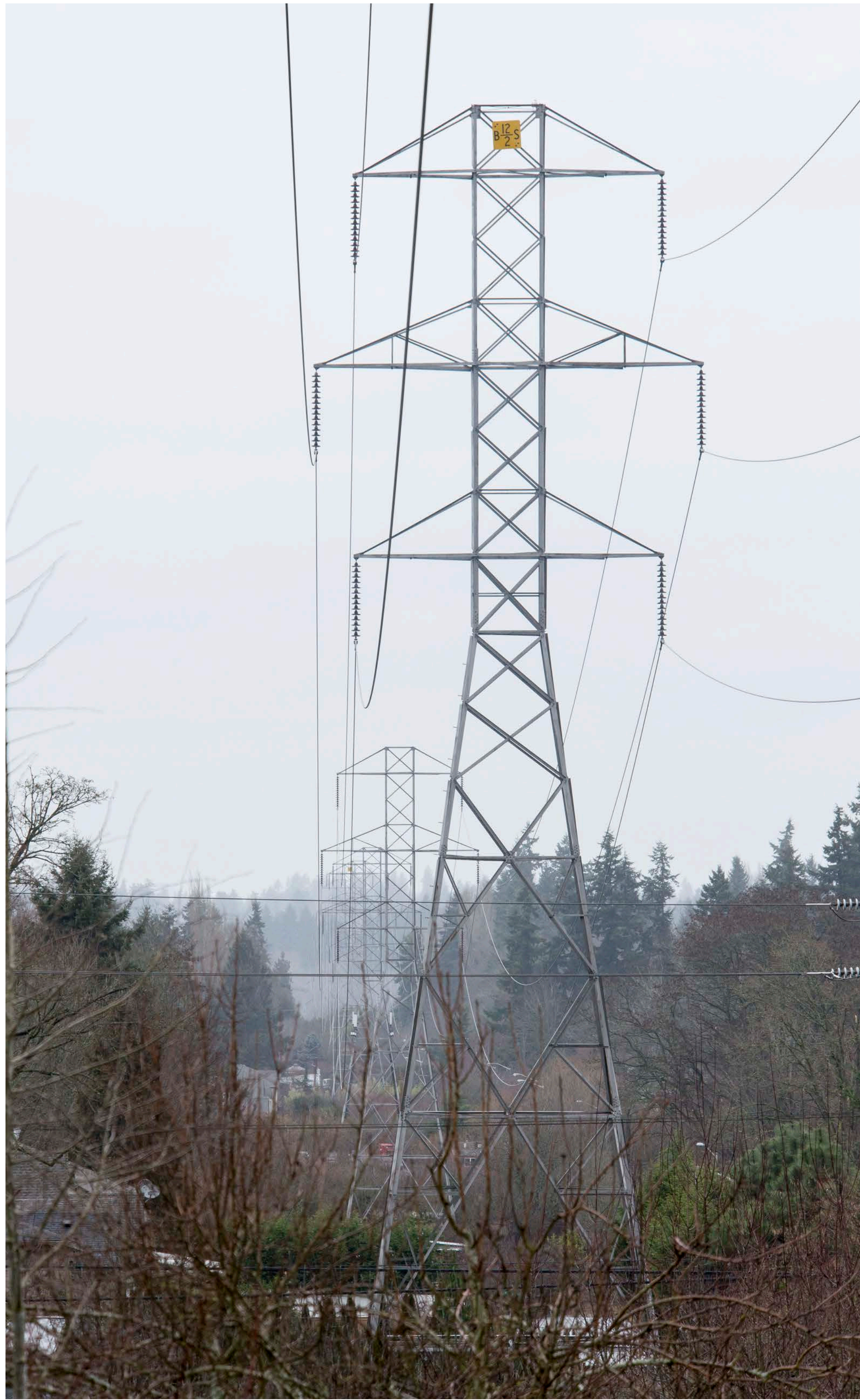
A Seattle City Light 230 kV transmission lines.
