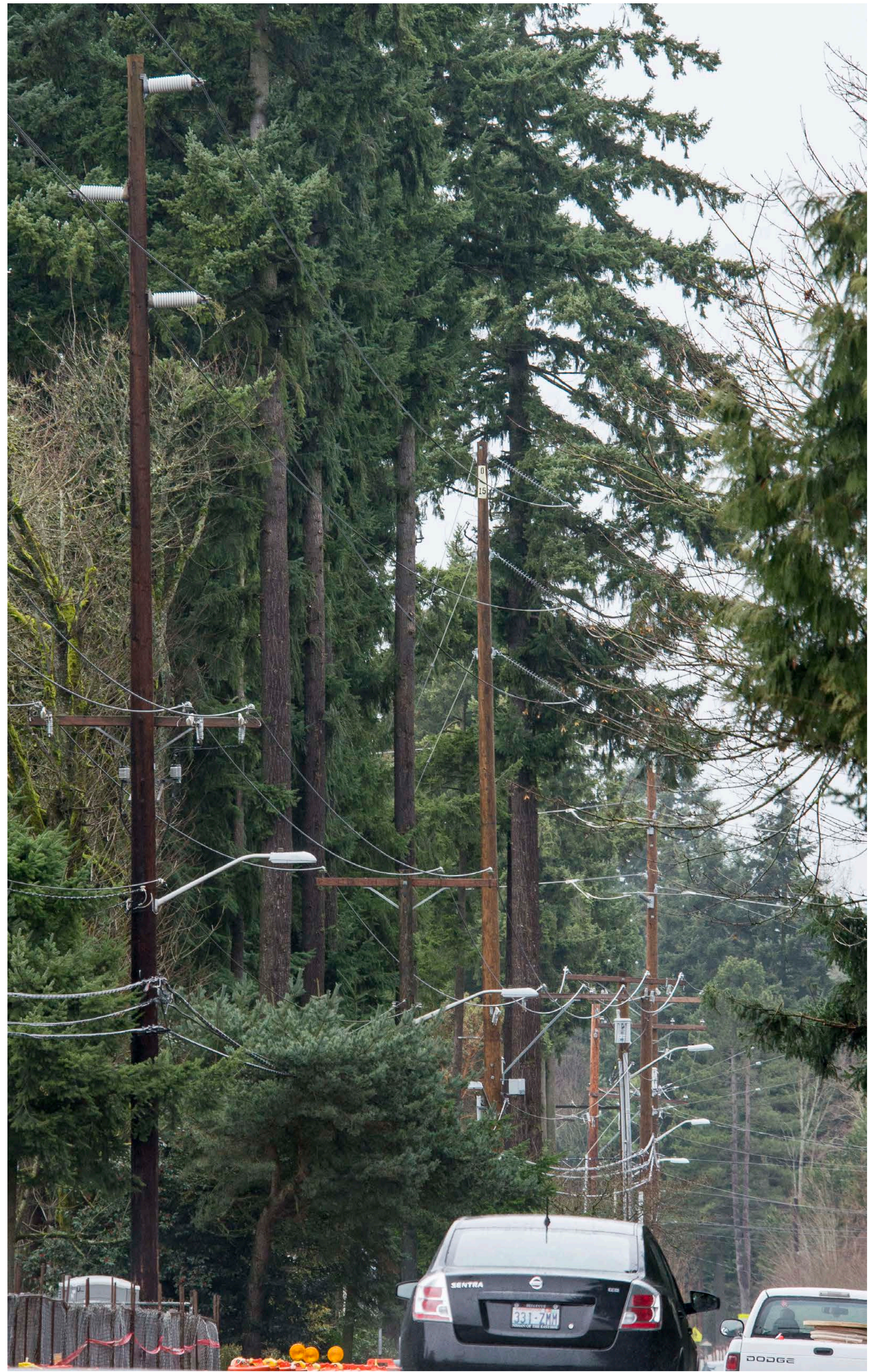
B 115 kV transmission lines with distribution underbuild. Proposed route segment B.
